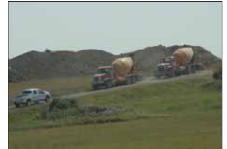
Cement trucks were a common site at the Prairie Winds wind farm site as crews poured concrete bases for the turbines.
