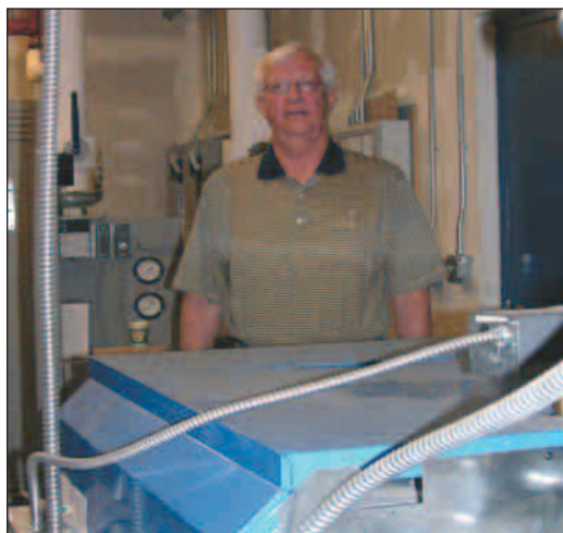
▶ John Klungtvedt likes the added comfort and safety provided by an electric boiler system while still recycling waste oil for heat. The new Farstad Oil shop is all-electric.
